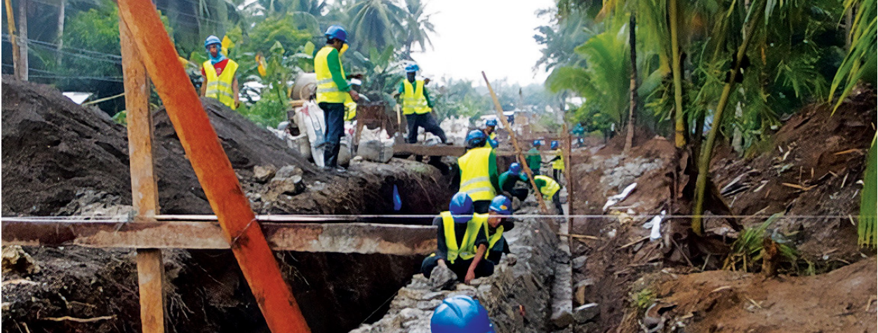
Construction of stone masonry walls for embankment protection along Samar Road in MCC's Compact with the Philippines.
