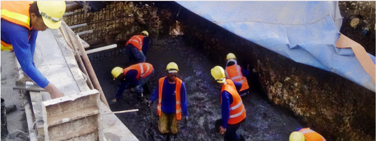
Construction of reinforced concrete box culverts to manage stormwater from increased rainfall intensity and reduce flooding on Samar Road and adjacent properties in MCC's Compact with the Philippines.
