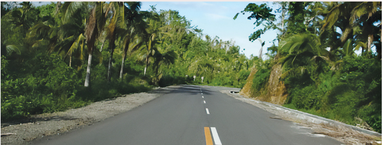
In MCC's Compact with the Philippines, Samar Road was designed for improved road safety and drainage to account for climate change while minimizing environmental and social impacts.
