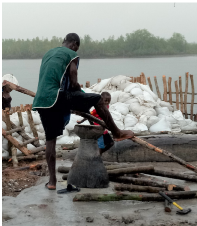
Workers building embankments to increase resilience to climate change in West Africa.
