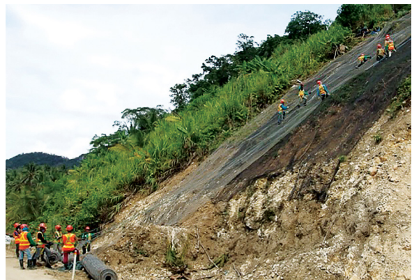
Slope stabilization using high-capacity, non-corrosive netting as part of climate-resilient design on the mountainous section of Samar Road between the towns of Wright and Taft in MCC’s Compact with the Philippines.
